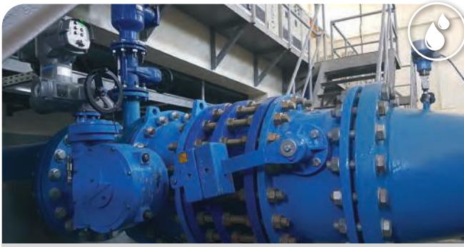
Station de pompage | Eau | OUGANDA Pumping station - Water - UGANDA
