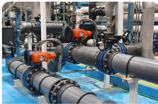
DESALINISATION | Eau | EMIRATS ARABES UNIS Desalination | Water | UAE
